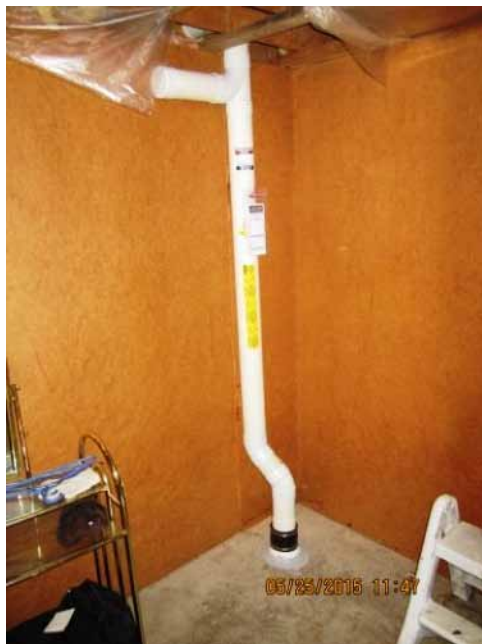
Figure 5. Radon Vent Pipe through Sub-slab
