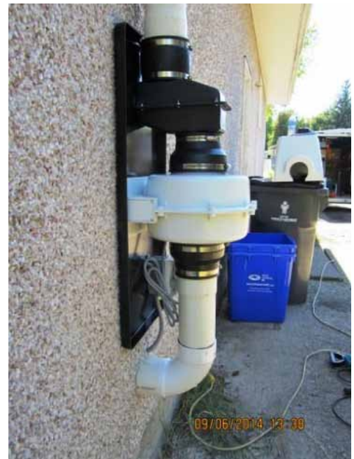
Figure 6. Radon Pipe Venting through Side Wall
